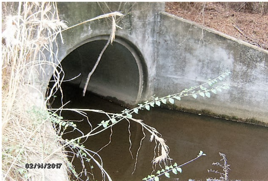
Figure B-8. View of the north side of the drainage culvert that underlies Moses Cook Road where sediment and surface water sampling associated with RI studies of Area 9100 were previously conducted.
