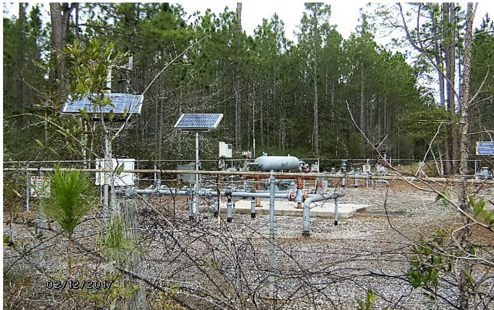
Figure B-3. View of the Gulf South Pipeline metering station just outside the NASA Fee Area northeast of Area A.
