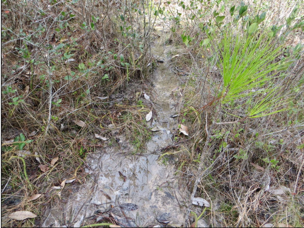
Figure 7. Water seeping out of the hillside above Turtleskin Creek in Parcel A.
