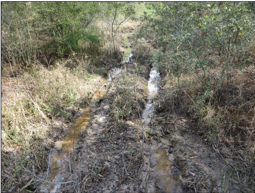
Figure 29. Road in Parcel A running through a very wet area.
